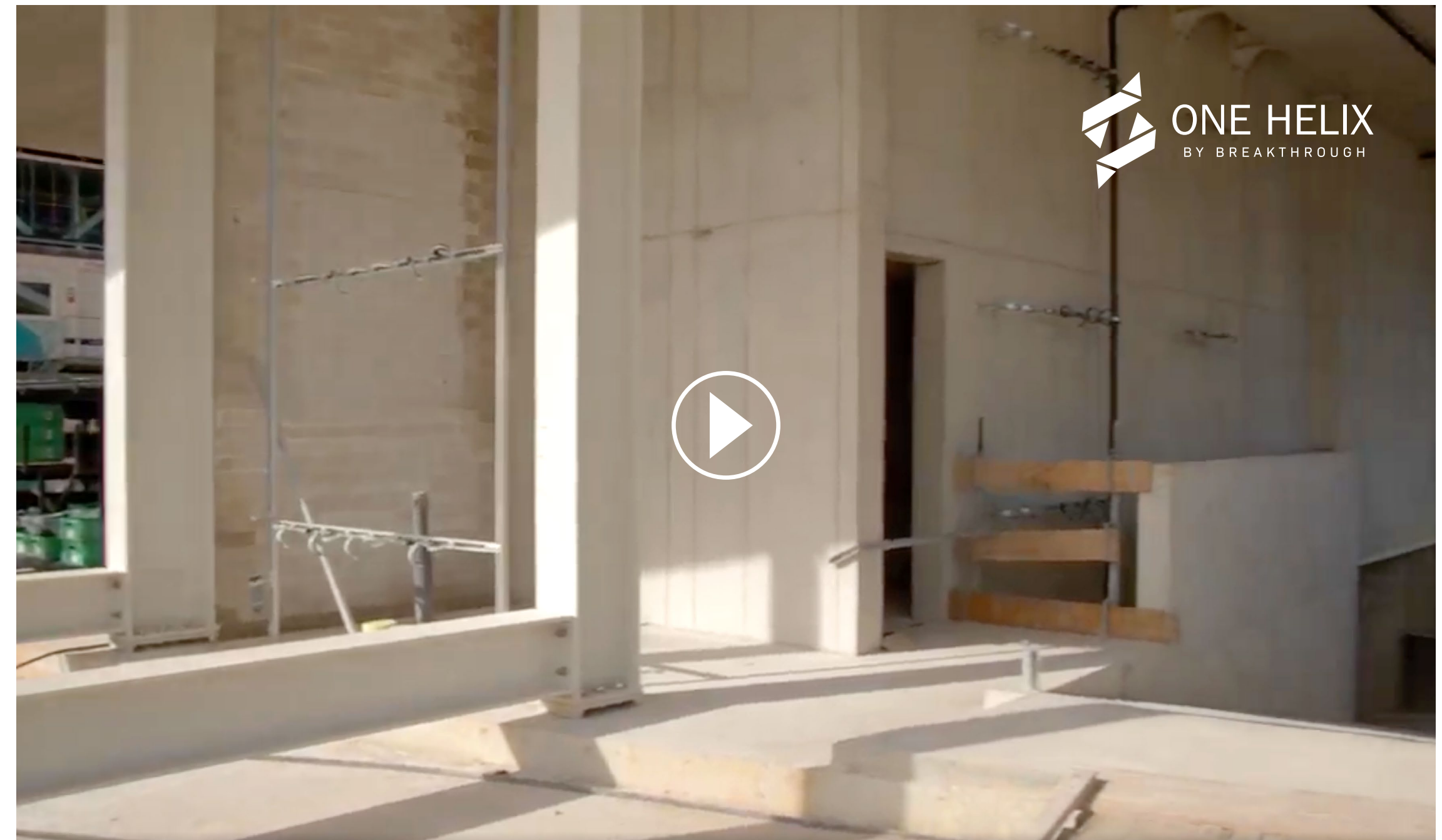
Construction walkthrough of One Helix demonstrating our innovative approach to delivering sustainability on this project. External link leading to LinkedIn.
